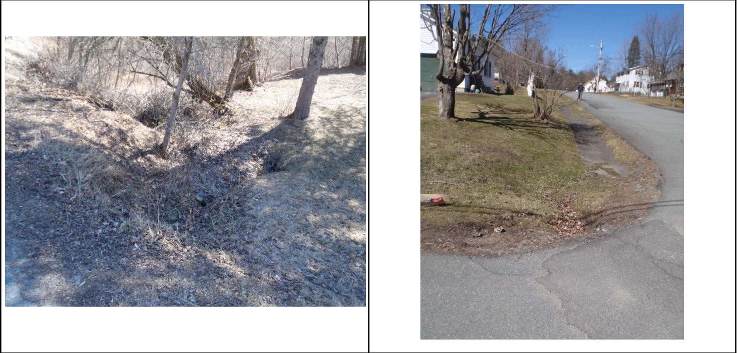
Photo 1: Gully erosion where Farmer Dr crosses unnamed tributary to the Passumpsic Photo 2. Paved swale along Waterman Circ. at intersection with Farmer Dr.
