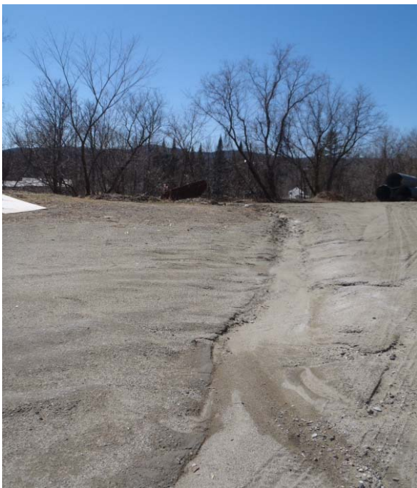
Photo 1. Gully erosion through Town Garage maintenance yard
